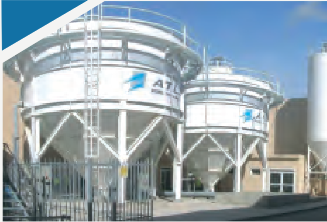
DRINKING WATER TREATMENT PLANT
