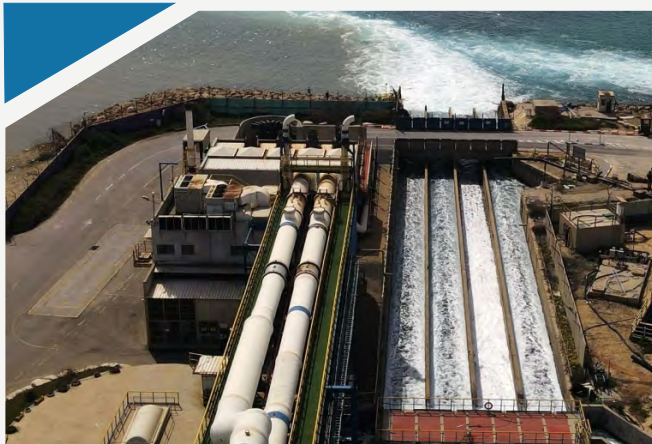
SEAWATER DESALINATION PLANT
